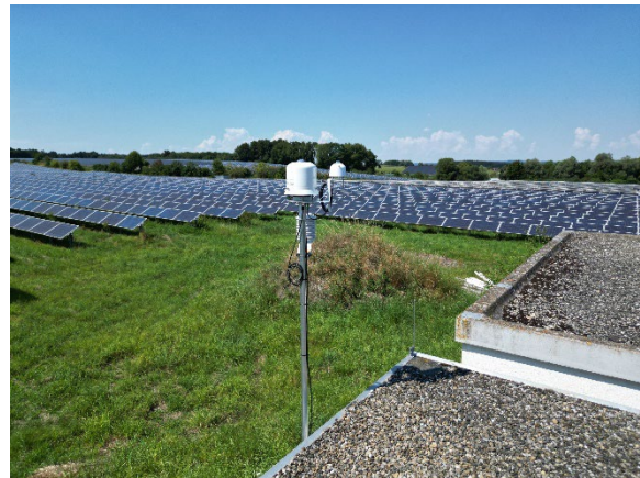
Figure 10: ASI 16/55 on the roof of a technical container at the Bittenwiesen I site. As in the previous figure, the pyranometer for measuring global radiation is visible here as well. The radiation shield with the temperature and humidity sensor is not visible due to the viewing angle.
