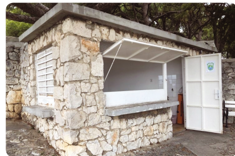
Figure 36: The initial state of kiosk, Prva Vidilica, Split
