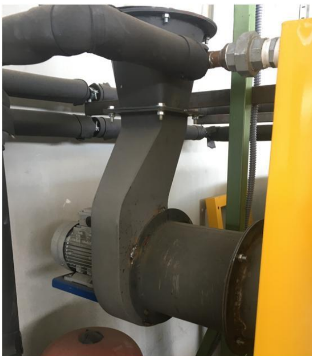
Figure 4.9 Exhaust gas ventilator installed in TK-25
