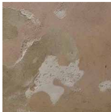
Figure 1: Overviews and details of salt efflorescences and moisture areas on granite and cement plaster covering the schist masonry
