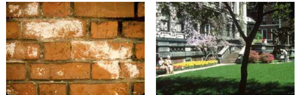
Figure 2: Detail of the brick wall showing the gypsum efflorescence formed on the parallel wall below grade to that seen in the garden at right.
