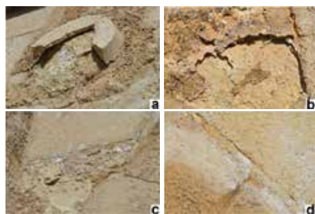
Figure 3: The damage forms on stone blocks. a) detachment of "artificial stone"; b) scaling and disaggregation of the original stone blocks; c-d) efflorescence on mortar joints and surface of artificial stone
