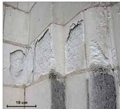
Figure 1: Example of spalling in tuffeau at the "Chateau de Chambord" (France) 3
