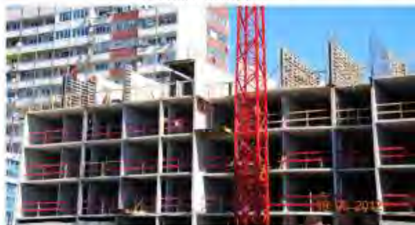
Varna. Construction of a residential building with a monolithic on-site cast concrete structure, 2013
