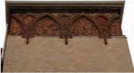
Sofia, 51, "6-th September" Str. Building Cooperative with masonry decorations, 1929, fragment, design by arch. Pantalei Tsvetkov and arch. Theodor Goranov.
