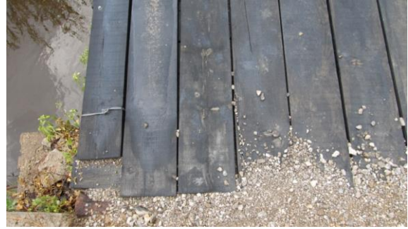
Figure 3: A bridge in the centre dyke that was repaired by Morsko Dobro (photo: Romy Durst)
