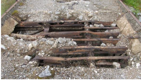
Figure 2: Ruinous bridge in the centre dyke of Tivat Salina (photo: Romy Durst)
