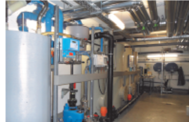
Photo 2: Greywater recycling combined with heat recovery. The combined system is placed in the basement where the building's heating system is also based, occupying an area of 9 \text{m}^2 (approx. 0.1 % of ground).
