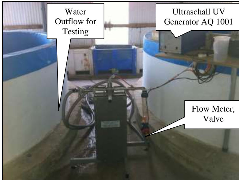
Fig. 1: The Ultraschall AQ 1000 US/UV reactor in the AquaVet wet – lab facility
