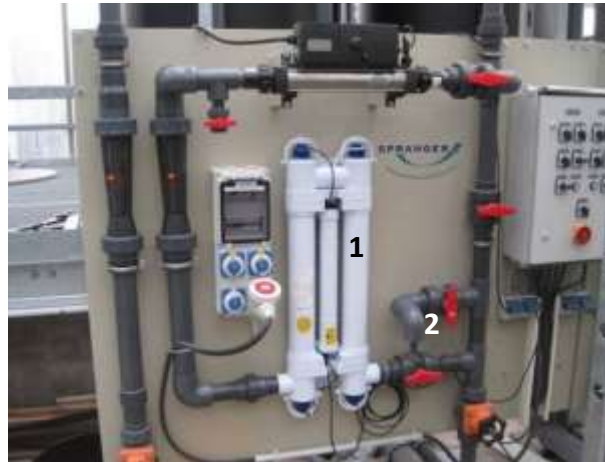
Fig. 4: UV-C reactor (1), optional connection to external reactors (2)
