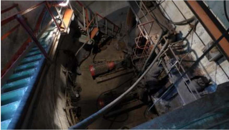
Pumpenstation in Chervonohrad
