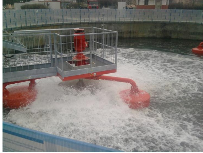
Figure 3. Aerobic sludge stabilization
