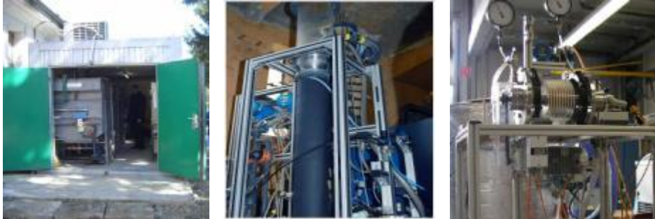
Figure 5: Various parts of the pilot plants in Romania.
