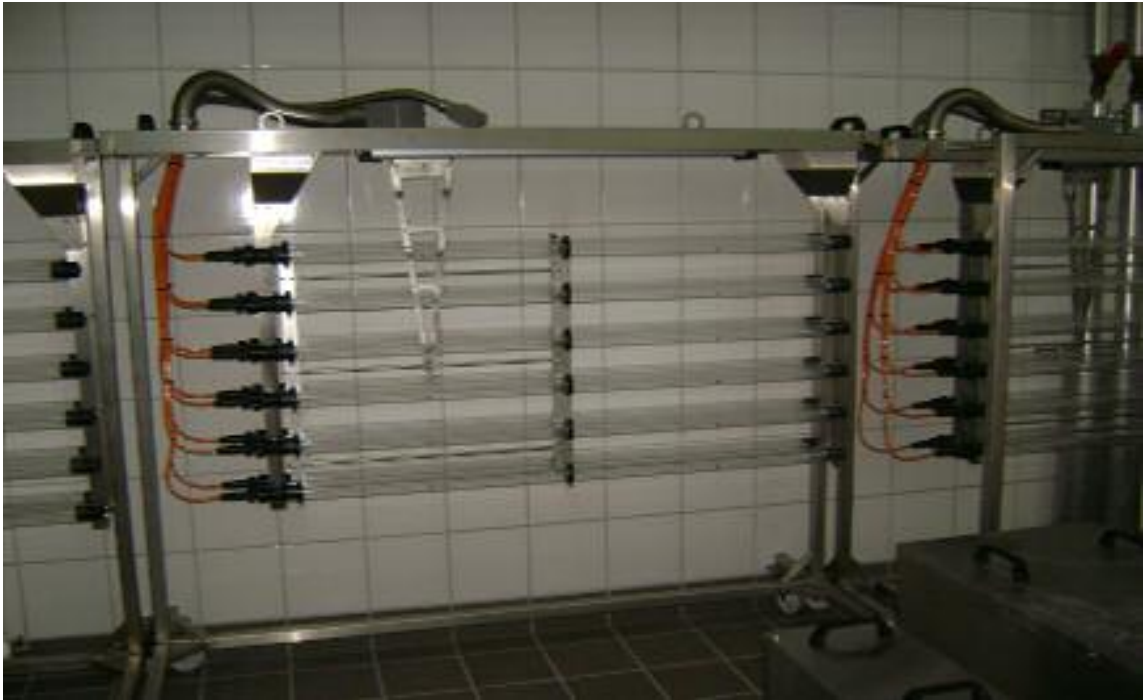
Photograph 8: Ultraviolet lamps for UV disinfection
