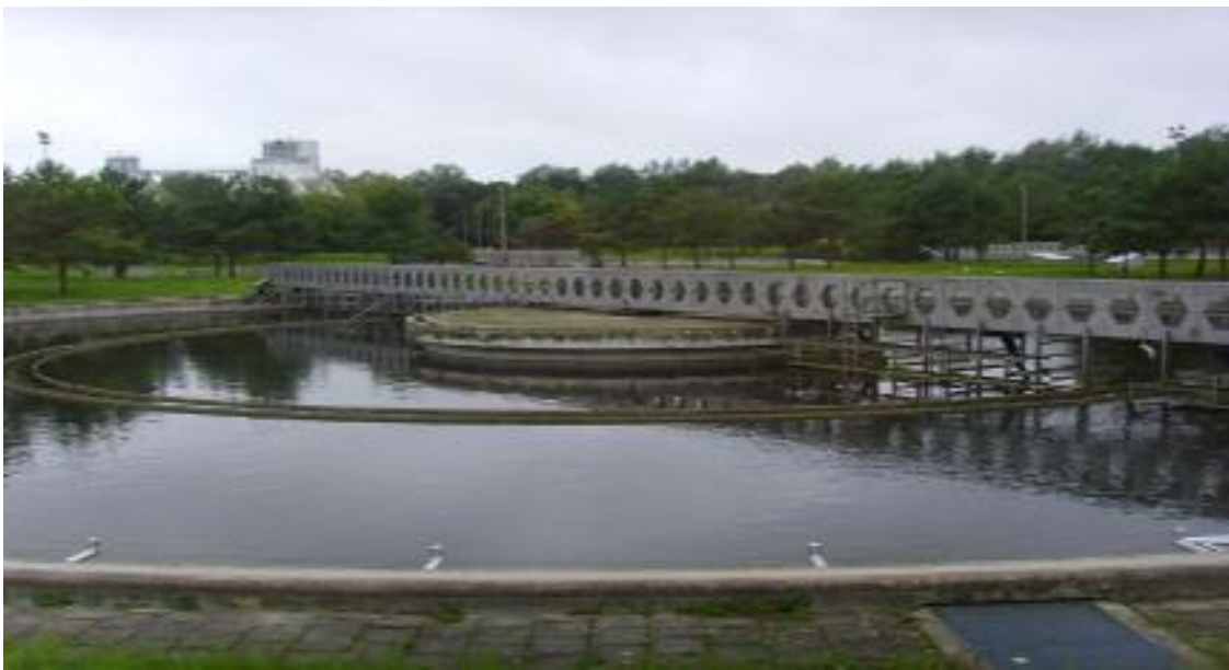
Photograph 6: Intermediate Sedimentation tank
