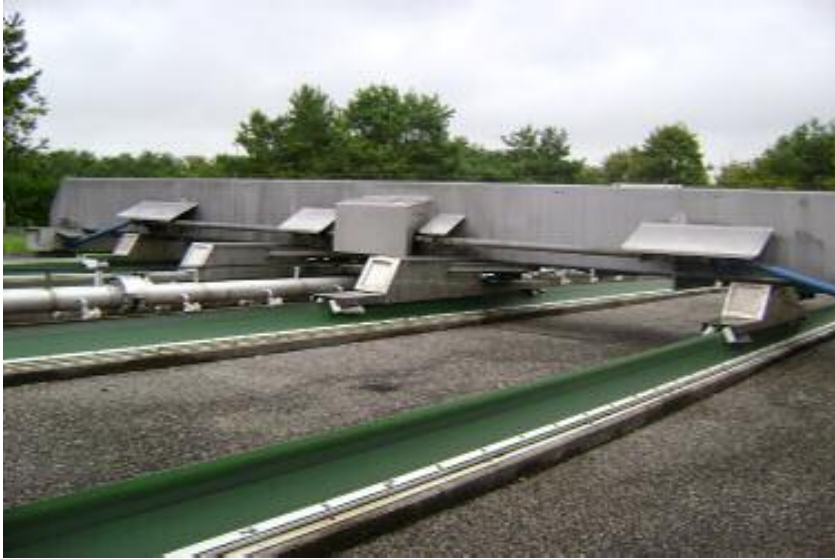
Photograph 4: Aerated Grit Chamber.
