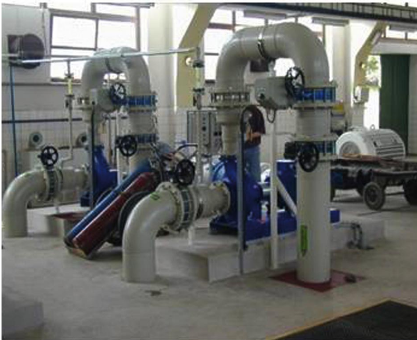
Figure 4. Pump station CHEVAK Cheb – water-processing unit Nebanice
