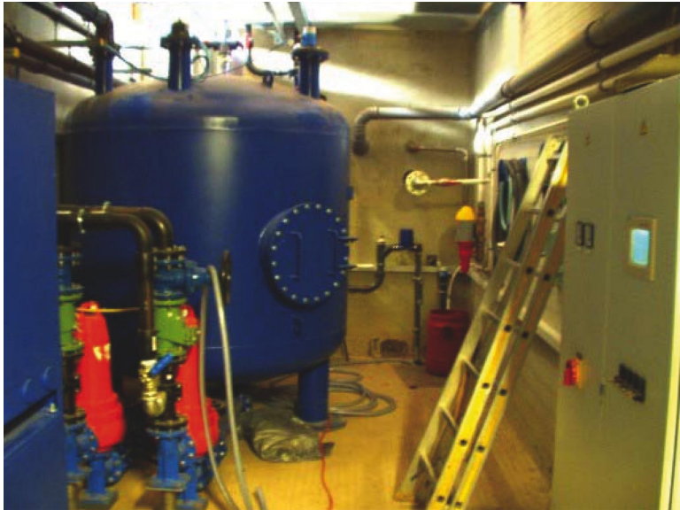
Figure 7. Vacuum station in the basement of the water house at the DEUS21 demonstration site in Knittlingen/Germany
