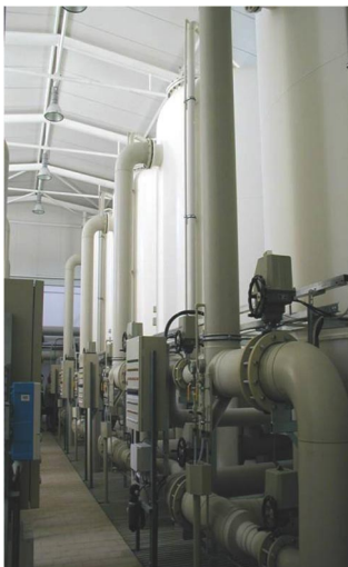
Figure 6. Biological filtration plant water-processing unit Nebanice
