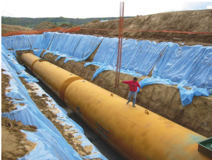
Figure 5. Rainwater storage tank during infrastructure provision works at the DEUS21 demonstration site in Knittlingen/Germany
