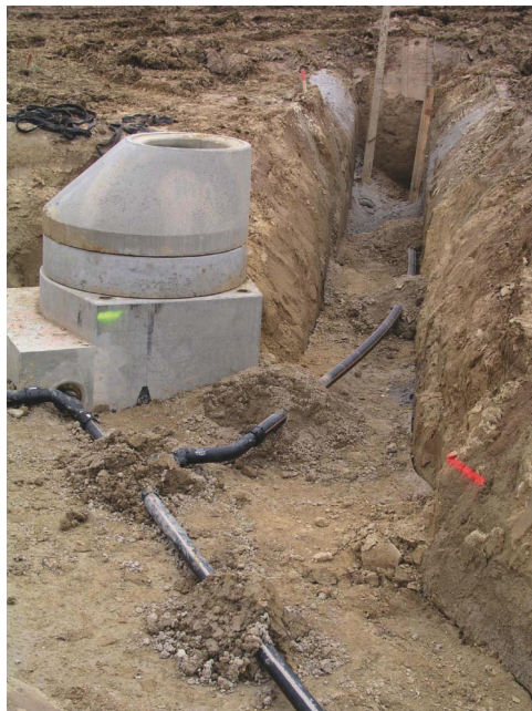
Figure 8. Vacuum sewer pipes during laying at the DEUS21 demonstration site in Knittlingen/Germany
